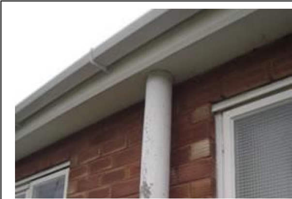
Asbestos cement drainage pipe (downpipe)
