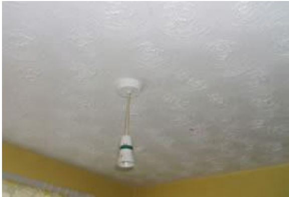
Asbestos containing ceiling tiles
